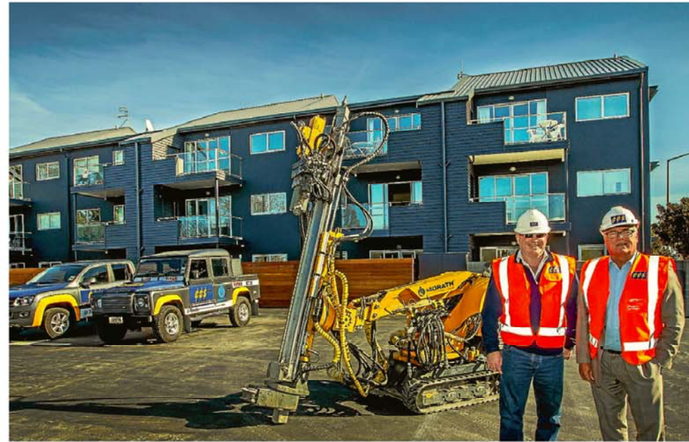
Core Civil Solutions director Wayne Tobeck and Colliers International managing director Hamish Doig outside the Salisbury St apartment complex many thought was a write-off but which was saved by new technology applied by CCS.
